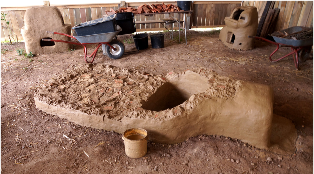
Abb. 4: Wannenofen GO-Borg-3 im Bau, links dahinter der fertig gestellte Kühlöfen KO-Borg-4 und rechts der fast fertige Hafenofen GO-Borg-4. – Building of the tank furnace GO-Borg-3, behind to the left the just finished annealing oven KO-Borg-4, and to the right the almost finished pot furnace GO-Borg-4.
